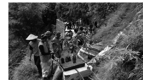
Resident-initiated forestation to prevent sediment-related disasters (Kelantan village at the foot of Mt. Merapi, Java, Indonesia).
